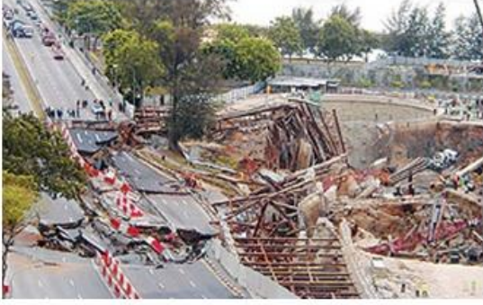
Singapore metro tunnel collapse
