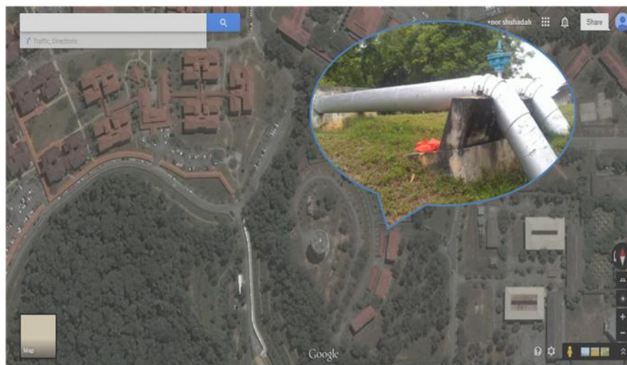
Figure 12: Pipeline from V2 water tank
