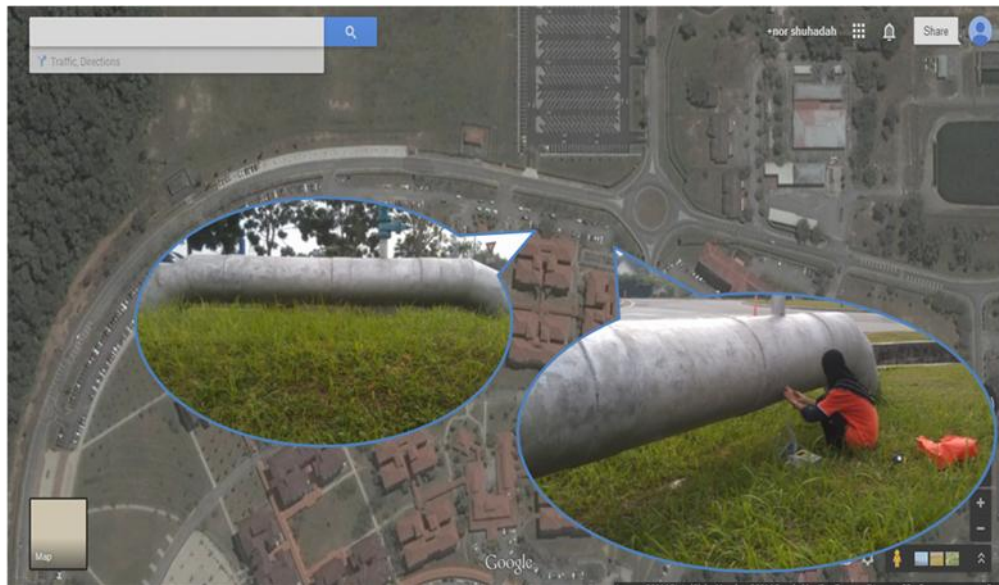
Figure 11: Pipeline opposite to V4
