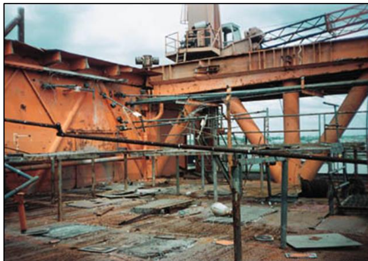
FIGURE 2.2 Condition of Ageing Offshore Platform
