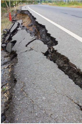
Figure 3: example of highway failure due to poor subgrade
