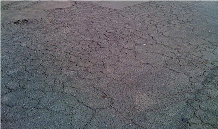
Figure 2: example of Alligator Cracking
