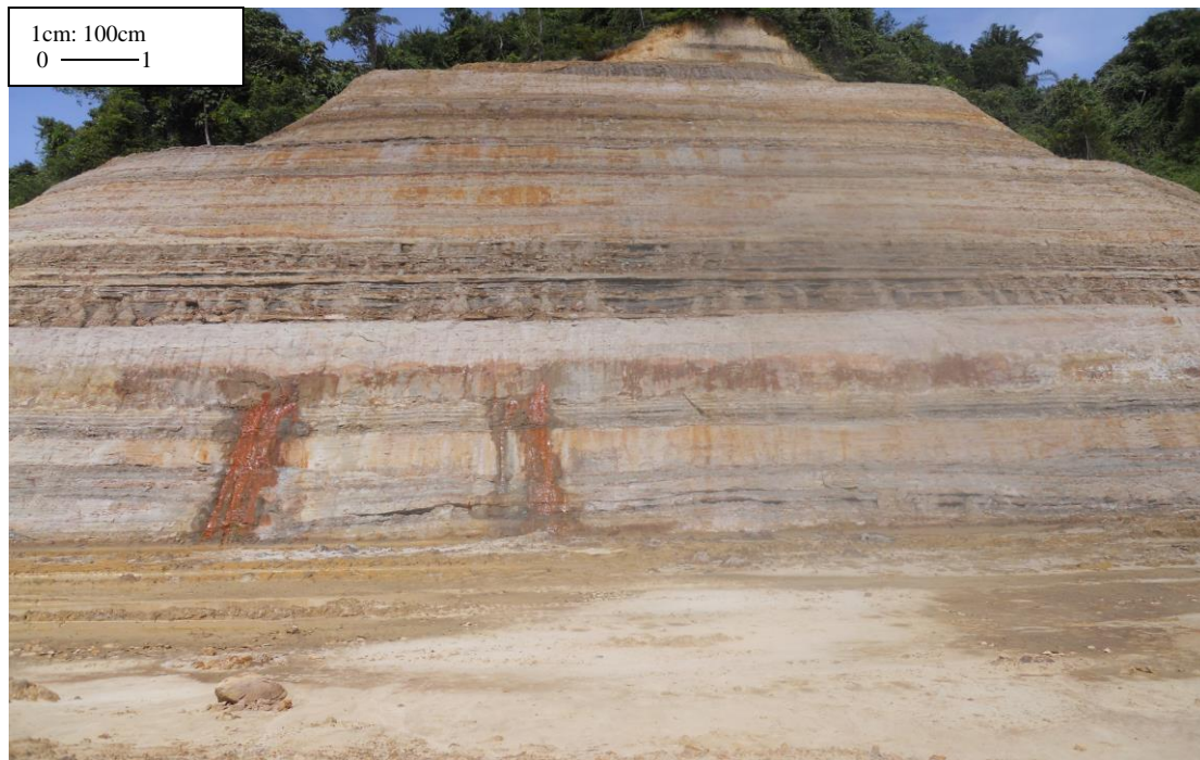
Figure 1: Outcrop of Hospital Road, Miri, Sarawak (Picture taken during field trip in January 2011)
