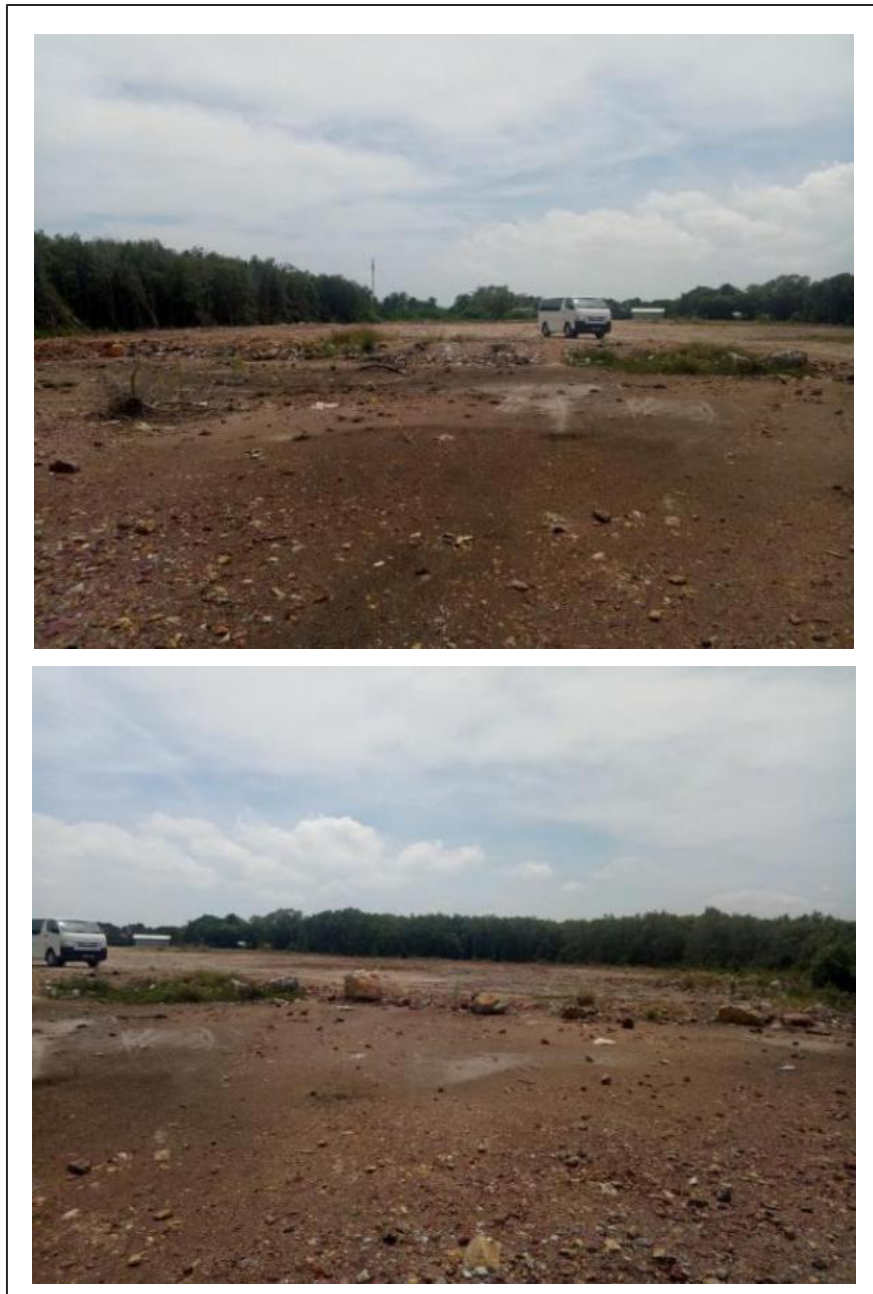
Figure 4.11: Clearance of mangroves in Kuala Kedah
