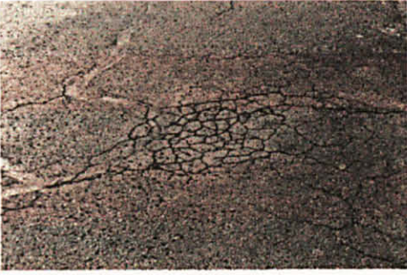
Figure A9: Alligator cracking
