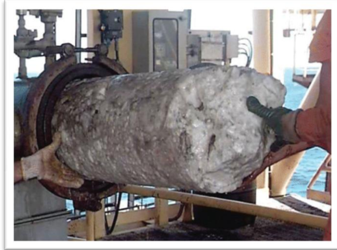
Figure 3: Example of Hydrate in Pipeline
