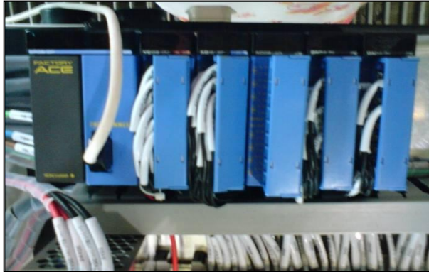
Figure 15: Programmable Logic Controller (PLC)
