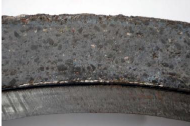
Figure 7: Typical pipeline cross section consisting of a steel pipe coated with asphalt enamel and concrete [22]
