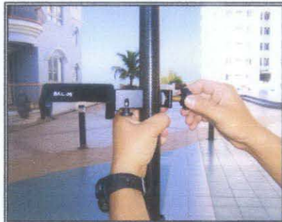
Figure 39: Bracket TSCe is installed at the upper part of the pole and make sure it is tighten
