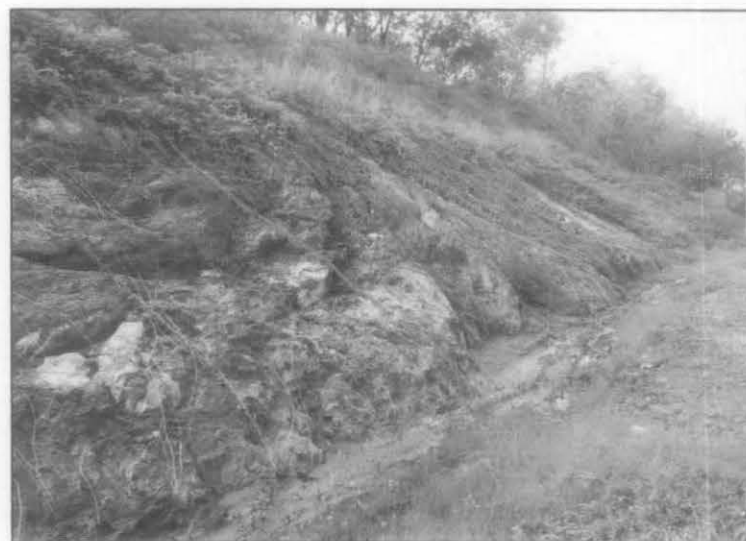
Figure 6: The location and condition of BG 3, near Kellie's Castle.
