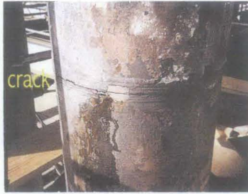
Figure 2.1: Crack/Creep failure on a gas pipe
