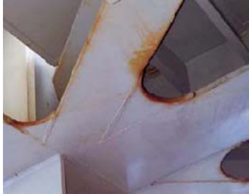
Figure A: Beam edge failure [10]
