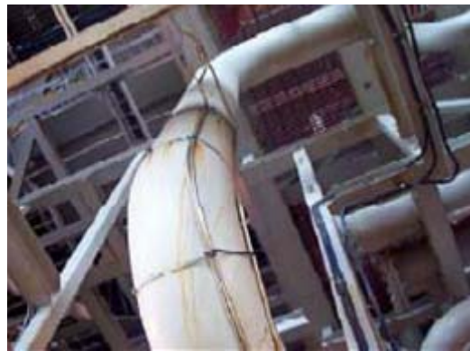
Figure B: Tubing on piping [10]
