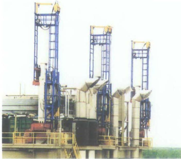
Figure 13: Active hydraulics accommodated in deck legs.
