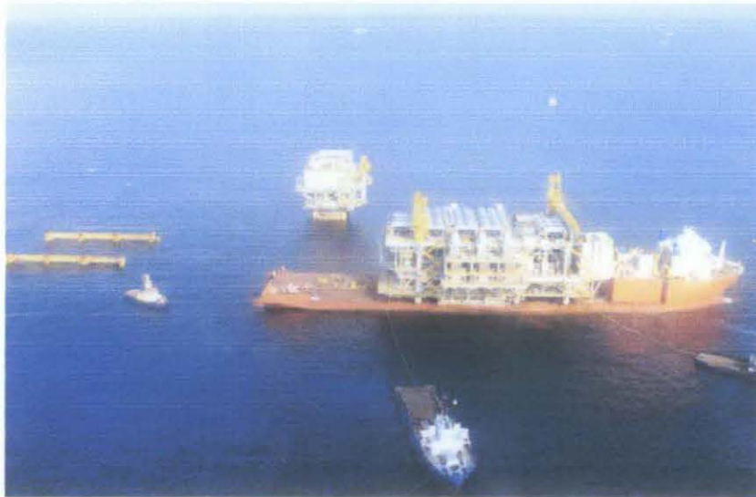
Figure 12: Self-propelled installation vessel Black marlin prior to entering the East Area Project GN Jacket
