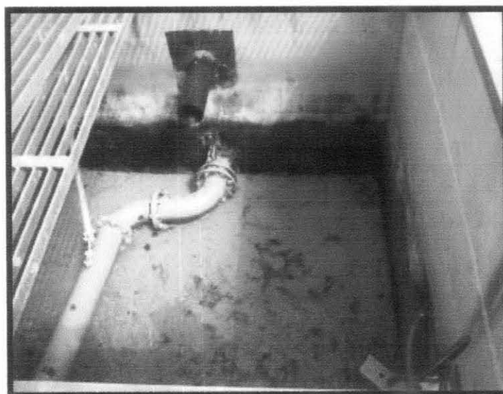
Figure 7 : Leachate after the Reed Bed Polishing Treatment
