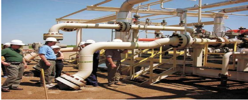
Figure F2: The Weyburn facilities where the main CO 2 pipeline comes from Beulah, North Dakota (Image courtesy of PTRC)
