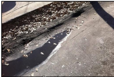
Figure 2.8.1: Rutting problem occurred on the pavement
