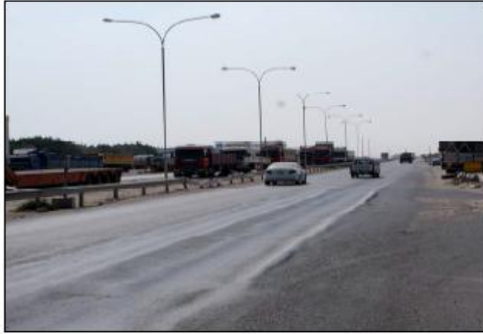
Permanent deformation in a road in Qatar
