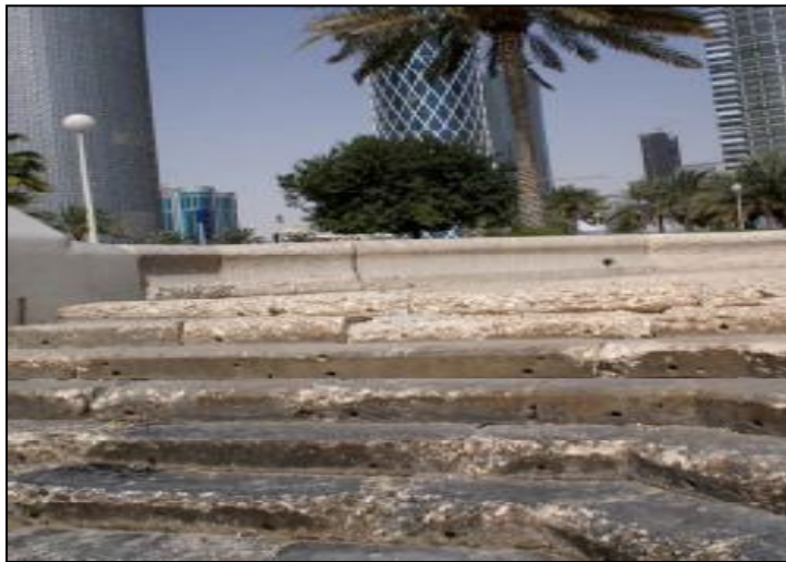
Portland concrete degradation from seawater in Qatar
