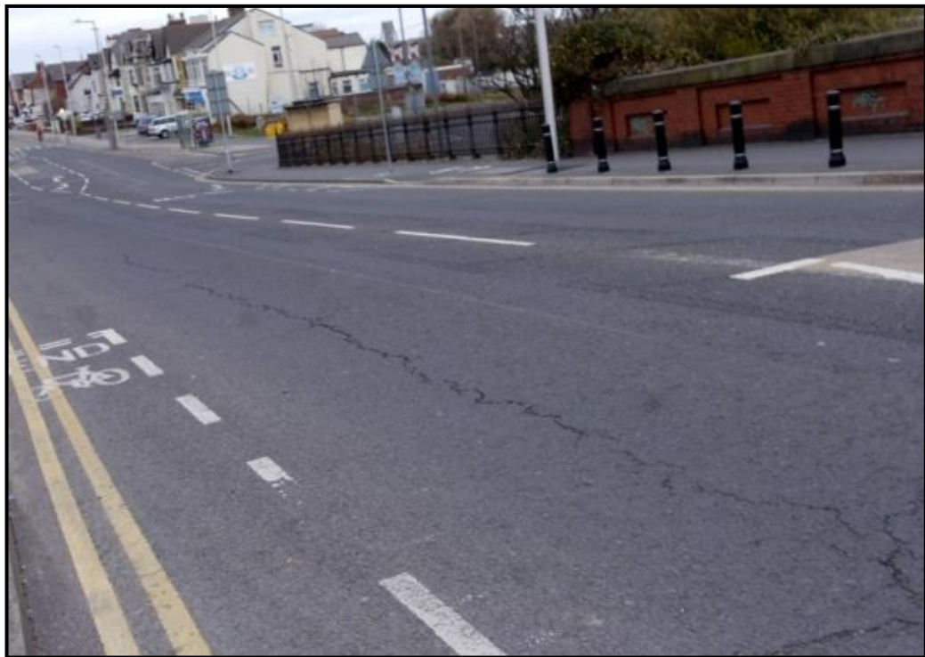
Figure 9: Damage have been caused by earthquake in UK
