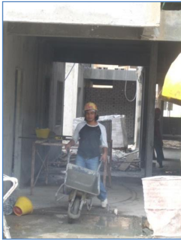
Figure 8: The worker didn't wear safety shoes
