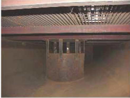
Figure 2.2: Typical Location of FAC at Bottom of Heater Shell
