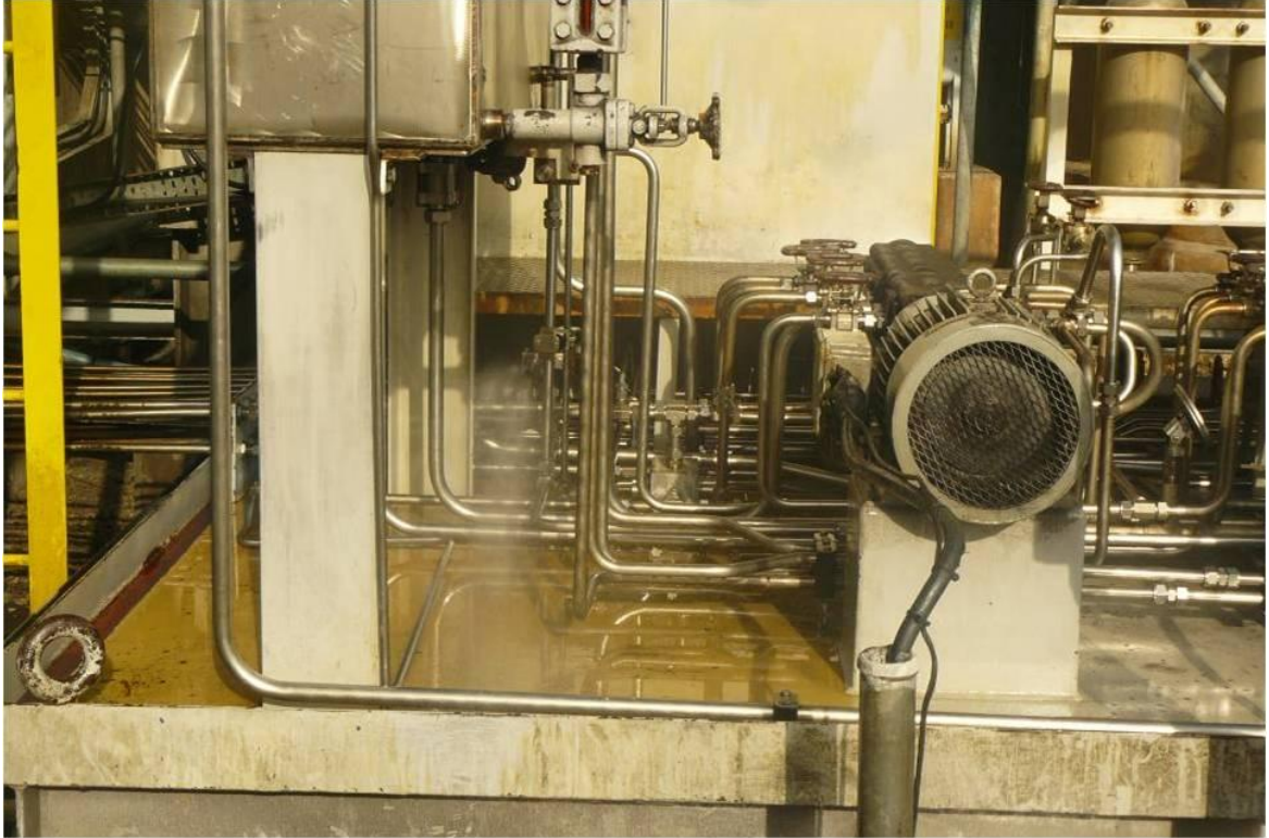
Appendix 2: Gas Generator lube oil console.
