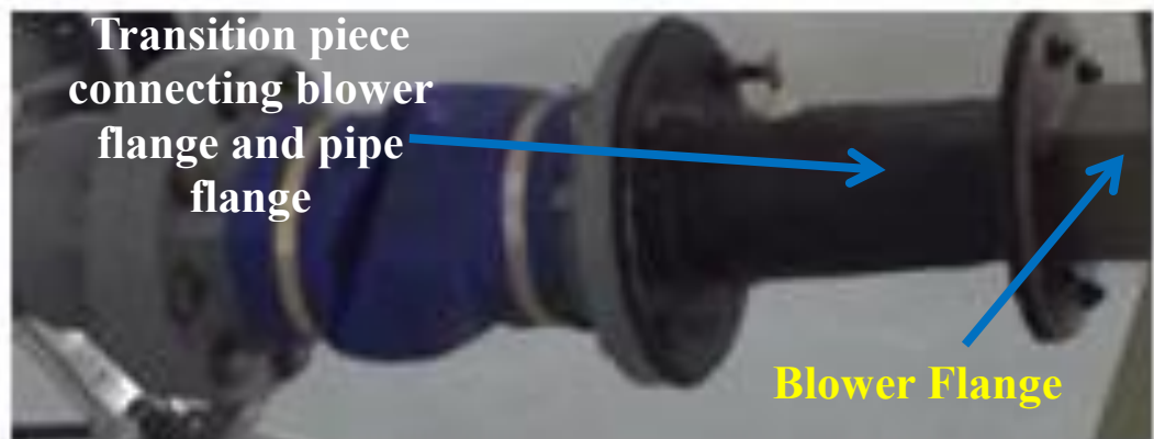
Figure 3.7: Blower flange and attachment
