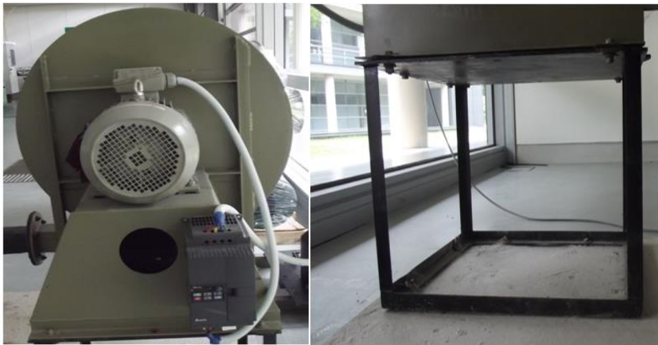
Figure 3.1: Blower and blower stand
