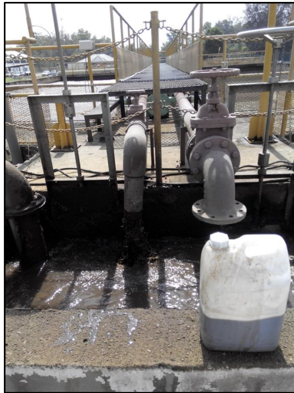
Figure 6: Return Activated Sludge at Anoxic Tank
