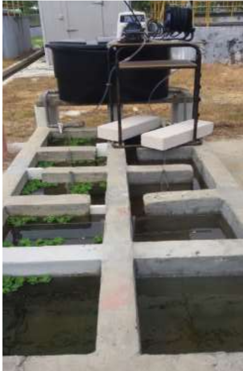
Figure 3.5 : Initial condition of water lettuce in Reactor 1 (day 1).
