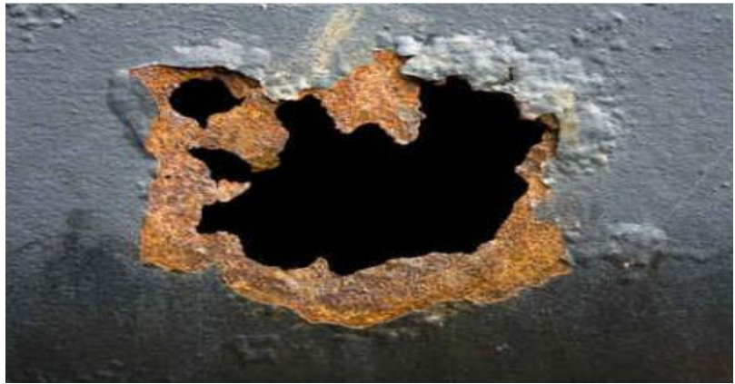
Figure 8. Corrosion on a typical Jacket Leg Surface
