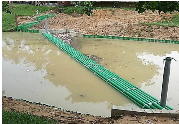
Figure 2.1: Floating Debris Trap
