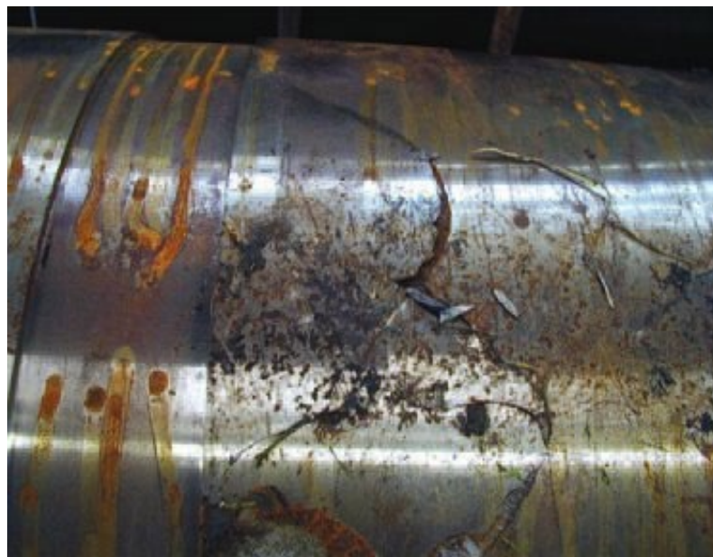
FIGURE 1.2 Pipeline Cracking Due to Embrittlement
