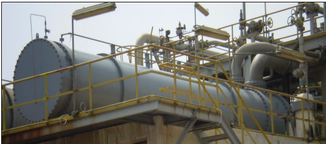
Figure 1 : Heat exchanger T-831
