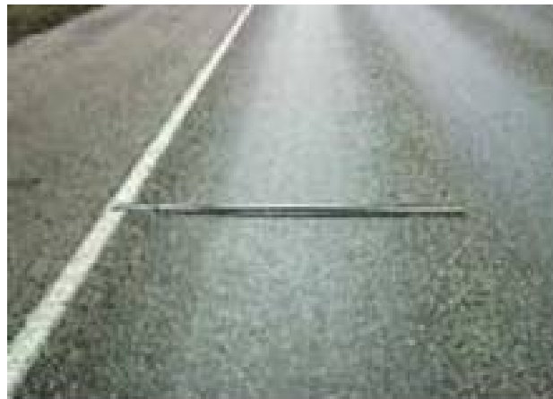
Figure 2-5 Rutting in pavement [52].
