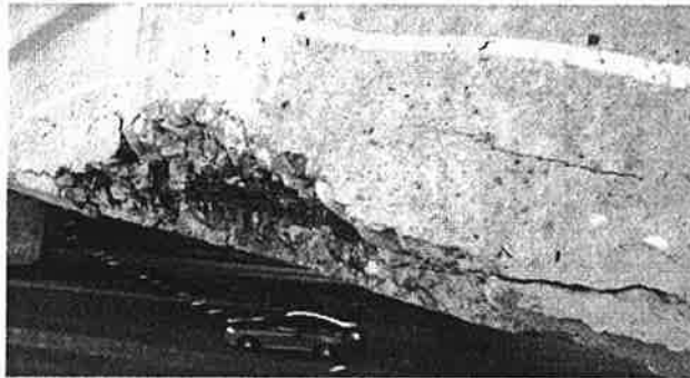
FIGURE Q4: DEGRADED CONCRETE
