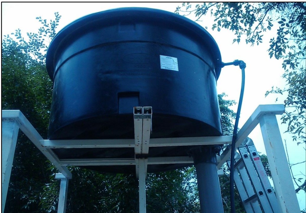
Figure 20: the water tank installed onsite
