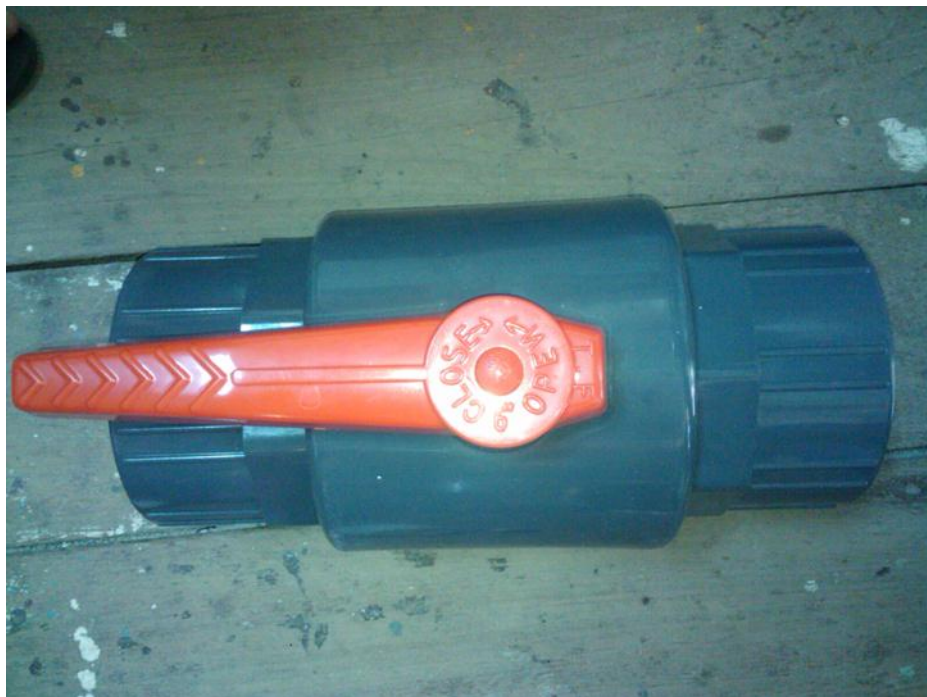
Figure 22: The manually-operated ball valve installed in the system
