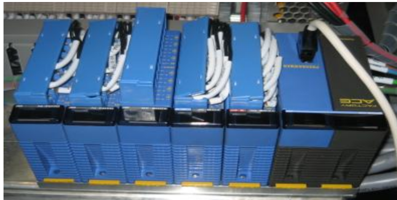
Figure 16: Yokogawa FA-M3 Controller
