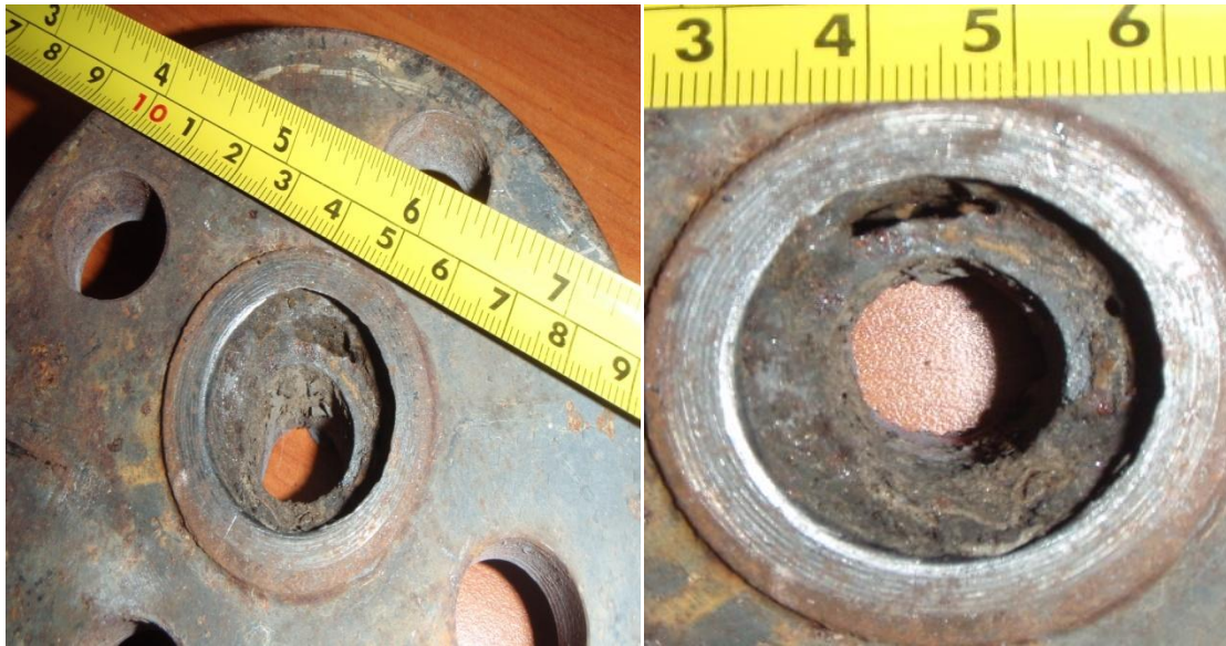
Figure A: Leak at 22-LG-04 Weld (Localized Corrosion)
