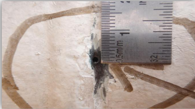
Figure B: Pin-hole leak at 6" KS-1 inlet piping to E-22-03 (d/s of 22-TG-05)
