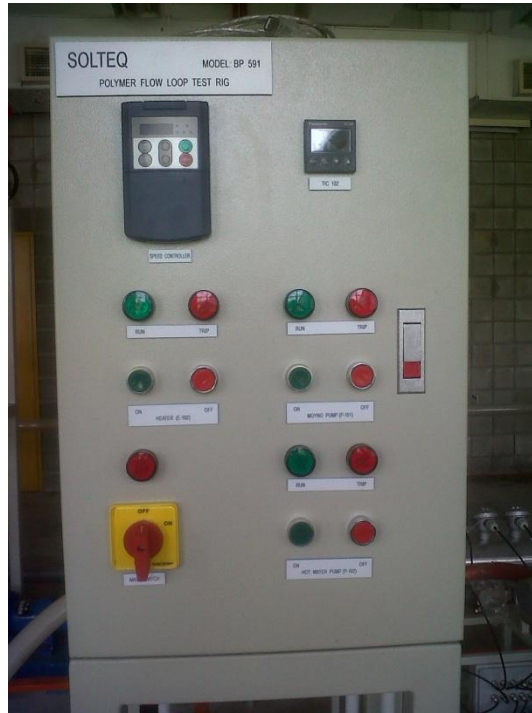
Figure 3-2: SOLTEQ Polymer flow loop system Control Panel
