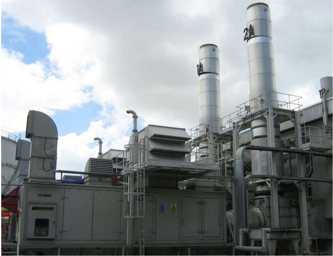
Figure 2.2 : Gas Turbine of GDC plant
