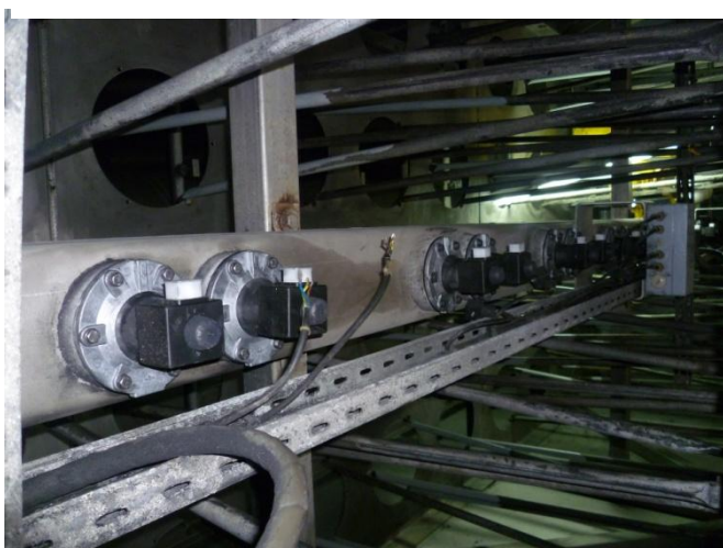
Figure 12: solenoid valve in the air filter house
