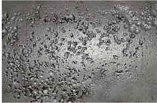
Deep pitting corrosion with some pits joining to form larger pits and interconnected pitting
