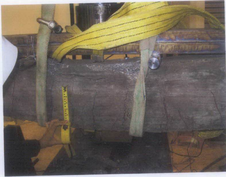
Crack occur at PFA 2 beam
