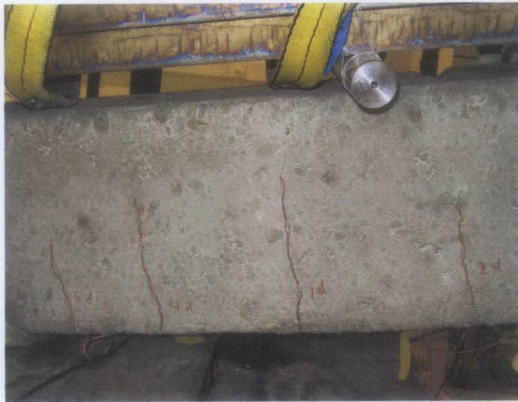
Crack occur at PFA1
