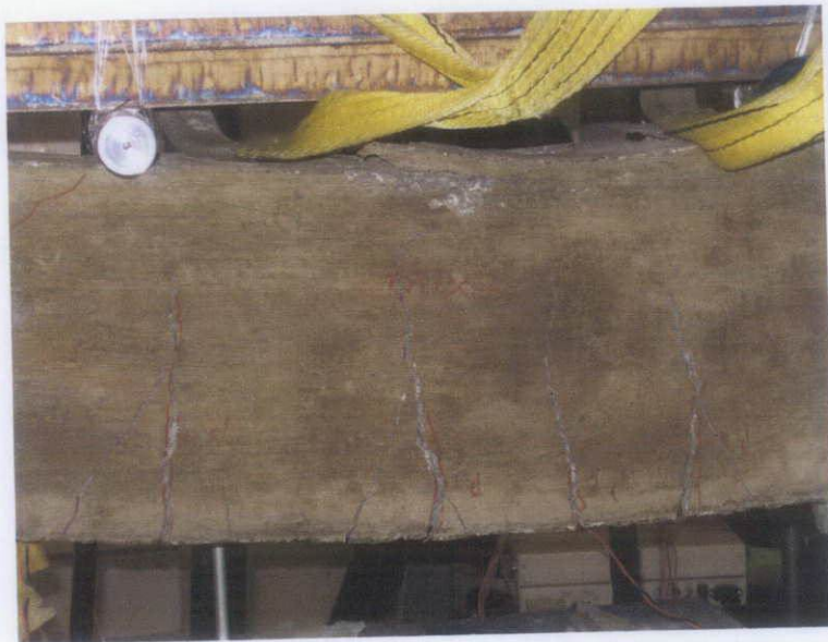
Crack occur at PFA3 beam
