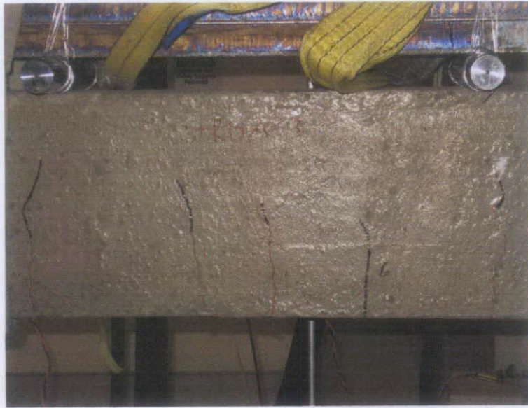
Crack occur at RHA 3
