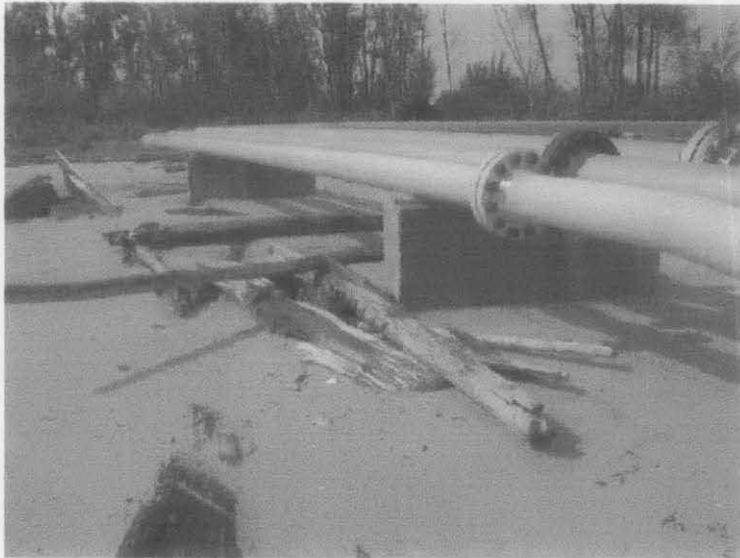
Figure 1.2 Pipelines support is in active zone
