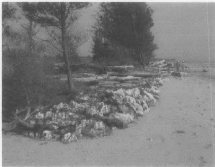
Figure 4.7 Gabion bund wall failures to protect pipelines
