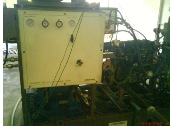
(k) Oil control panel
