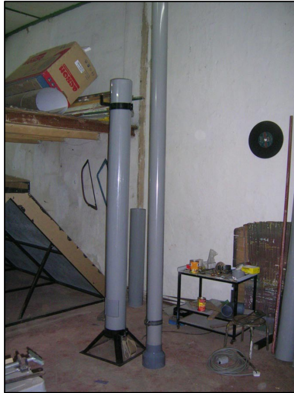
Figure 4.7 PVC Pipe Functioned as the Chimney
