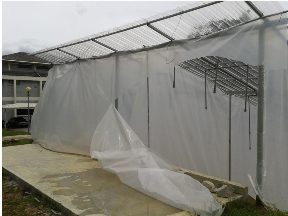
Figure 18: The top part has been ripped off due to heavy storm
