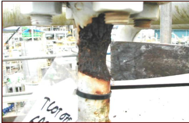
Small Bore Piping Failure at Air Fin Cooler (AFC)
