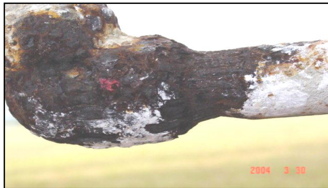
Internal erosion and external corrosion
