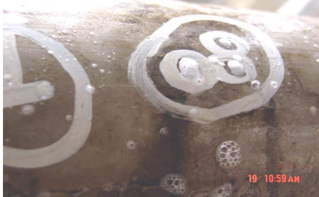
Chloride Stress Corrosion Cracking - leak spots at stainless steel pipe
