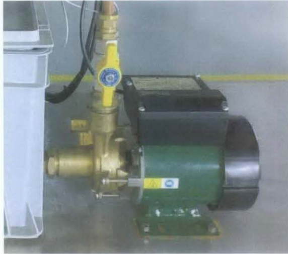
Figure 18: Lab water chiller pump
