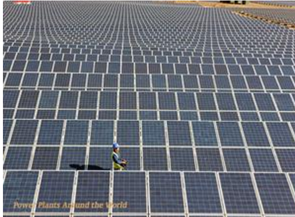
Figure 6 : Arnedo Solar Power Plant [10].
