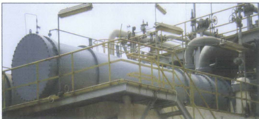
Figure 1 : Heat exchanger T-831
